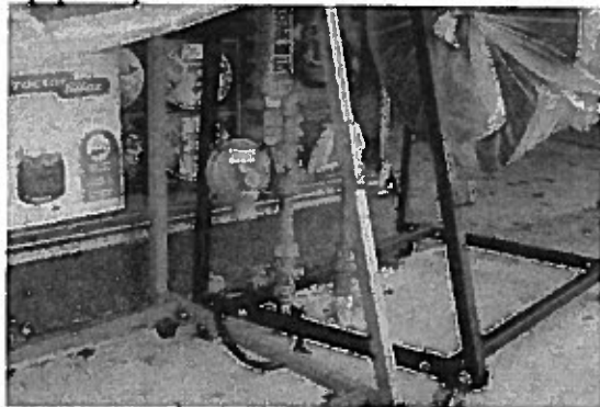
400 Block of 7 th St. 2011 Installation. Regulator used as security anchor.
