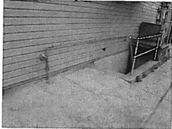
1000 Block of Chew St. 2012 Installation. Unprotected with excessive exposed piping likely to be utilized as a handrail.
