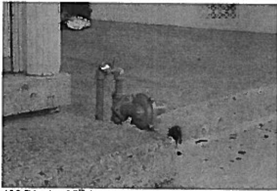
400 Block of 7 th Street 2011 Installation. Regulator presents a clear tripping hazard.
