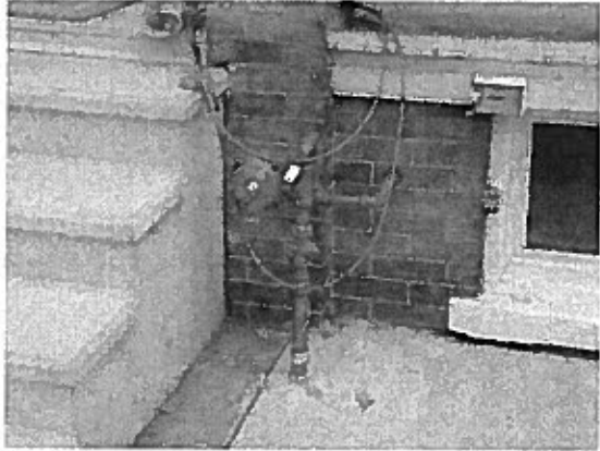
1600 Block of Turner St. 2011 Installation. Close proximity to stairs and regular foot traffic with no available options to hide or protect equipment.
