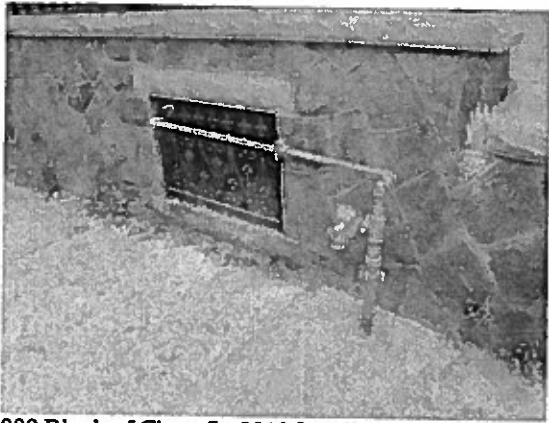
800 Block of Chew St. 2012 Installation. Unprotected with excessive exposed piping.
