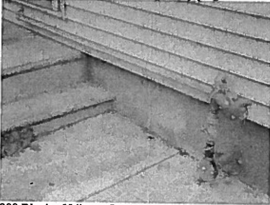
900 Block of Liberty St. 2011 Installation. Unprotected with excessive exposed piping terminating under center of front door.
