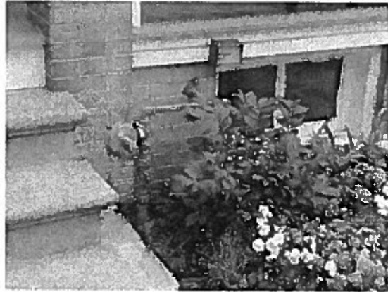
1600 Block of Turner St. 2011 Installation. Excessive exposed piping that is not consistent with other installations on the block.
